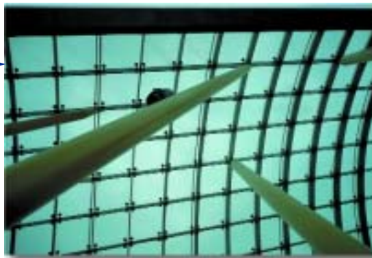
Bolted glazing system for the Shed Halle in St. Polten, Austria, seen from the inside
